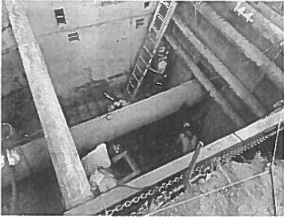
The Contractor finishes installment of rebar for concrete pad in Flowmeter Vault.
