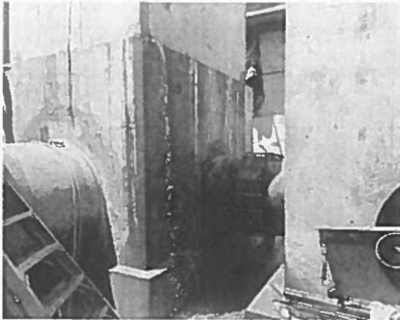
Large leak coming from Northeast corner of Diversion Box #2.
