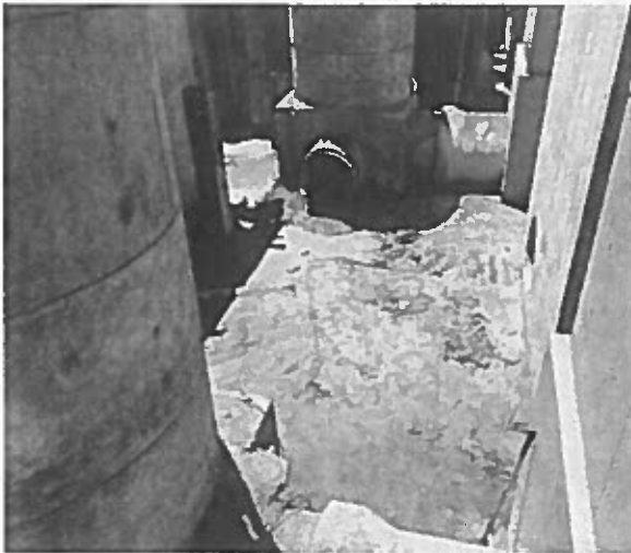
Slurry is poured into the excavation up to the bottom of the pipe penetrations.
