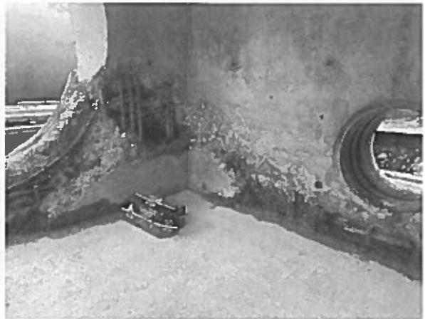
Inner formwork was removed from the bar screen structure and revealed significant honeycombing at penetrations. There was inadequate vibration around and below the penetrations: the Contractor advised that the vibrator became stuck at one point.
