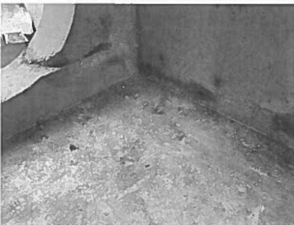
Honeycombing was patched with Sikacrete grout.
