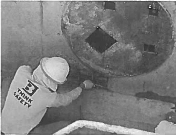
Outer formwork was removed from the bar screen structure and revealed honeycombing at its base.
